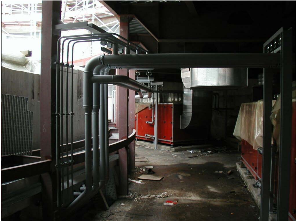
Fig. 3. Inside the GTC dome. Many complicated systems are required for the operation of the GTC. Some of the cooling subsystems are seen here.
