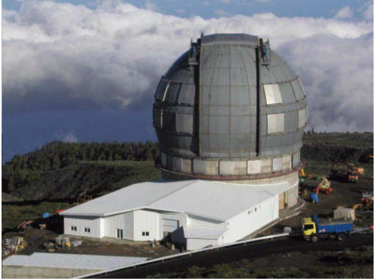
Fig. 2. Current view of the building site. Note that both the dome and building are nearly completed.
