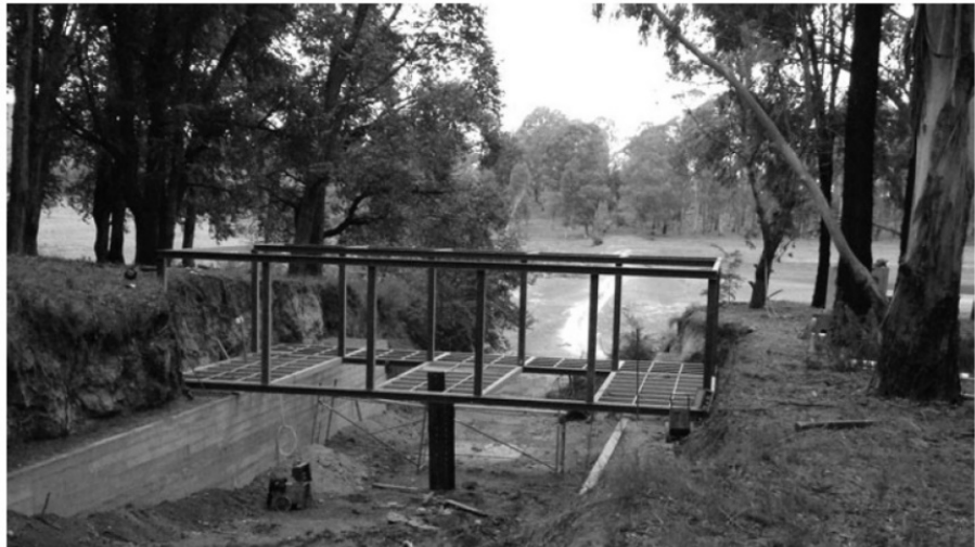
Figure 26: Assembly of a Vierendeel truss. Pabellón. (Source: Ferrer & Alarcia, 2014) This constructive outline allows for a definitive solution — diaphanous and free
