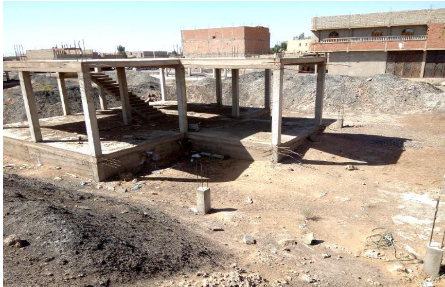
Figure 12: Housing developments near slag heaps and above underground mining tunnels.
