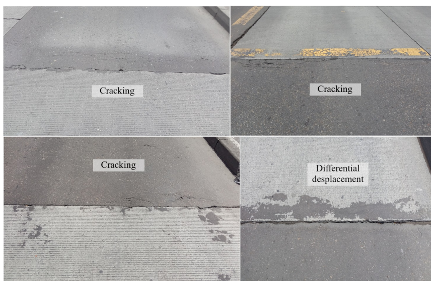
FIGURE 1. Distresses in direct ACP-PCCP transitions
