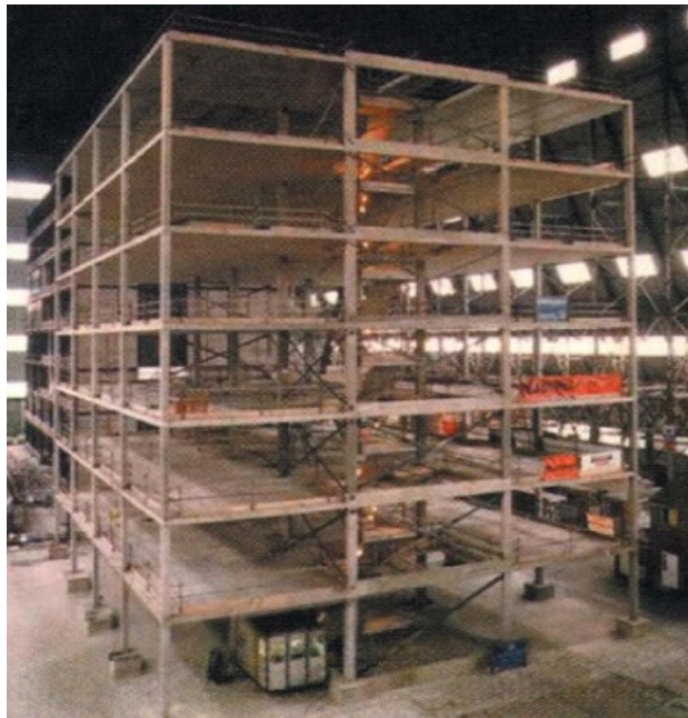
FIGURE 16 Perspective of the reinforced concrete prototype structure designed for the Cardington fire simulation experiment Chana & Price, 2003
