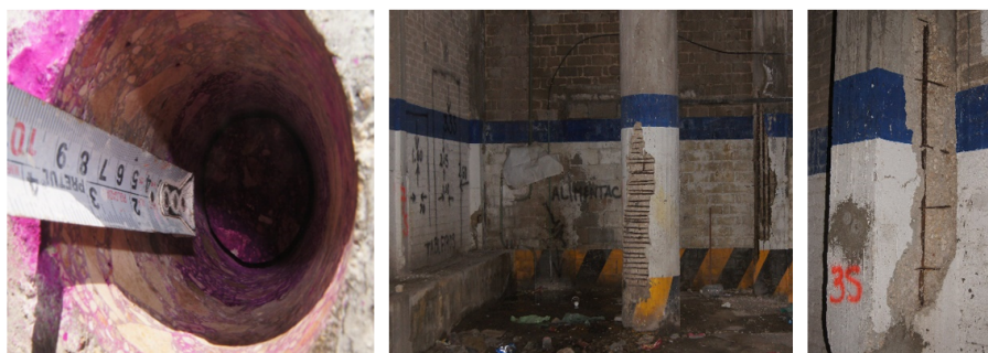
FIGURE 3 Carbonation and detachment of concrete.
