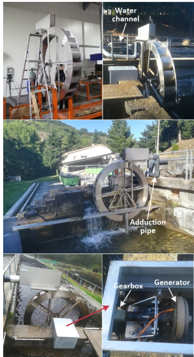
Figure 7 Stainless steel overshot waterwheel installed in the fish tank
