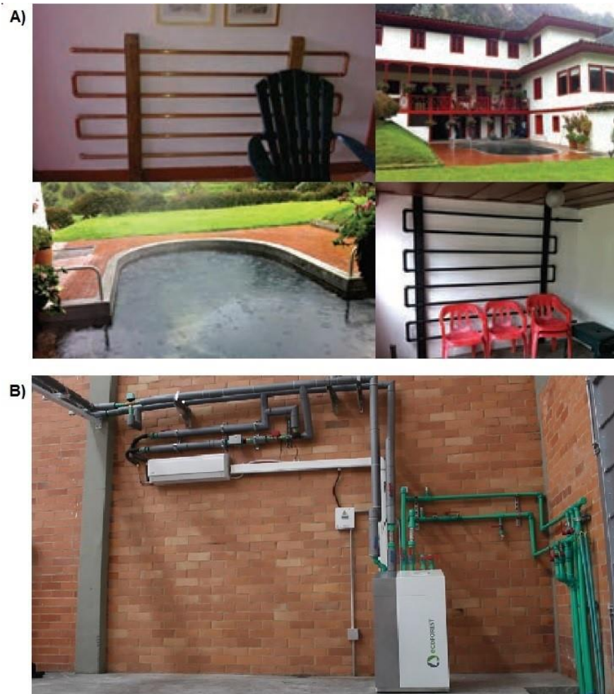
Figure 4. A) Use of geothermal heating at Hacienda La Quinta near the NRV geothermal area. B) Cold room with a geothermal heat pump pilot project developed in Bogotá by SAGG SAS
