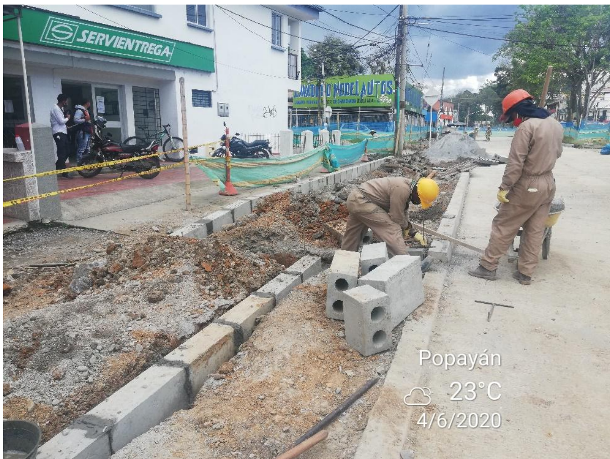
Figure 7. Issue identified regarding surface drainage.
