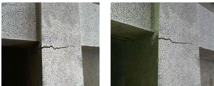
Figure 11. Cracking under concrete beams. Source: [1]
