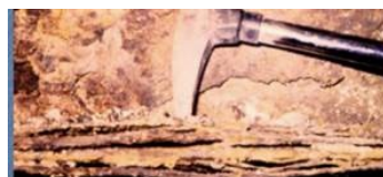
FIGURE 6. Exfoliation corrosion in a water treatment plant.
