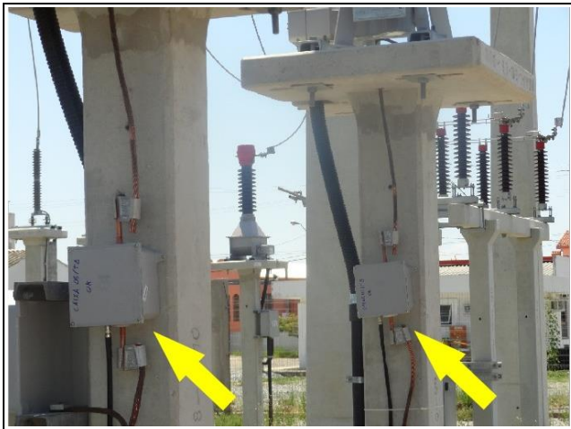
Figure 3. Enclosures containing current sensors and surge protectors installed at the grounding cables of CTs.
